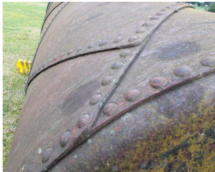
The workmanship of the diagonally riveted joints is amazing so catches everyone’s attention
