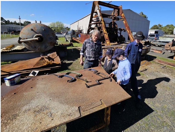
← The old heavily corroded floor plate laid over the new one to check position of holes and cut outs . It was so buckled it had to be pulled down with G clamps and through bolts by the boys . Greg pic
